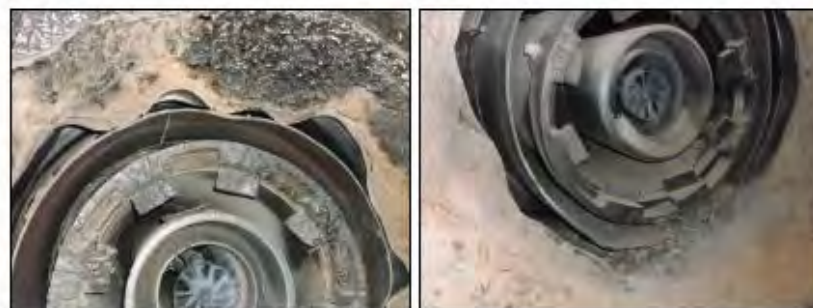
Figure 3: Rugeley existing burners showing extreme thermal damage and slagging
